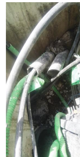
Figure 2: Fiber loose cable inside the PEHD tube (Courtesy of Fibrea-Covage)
